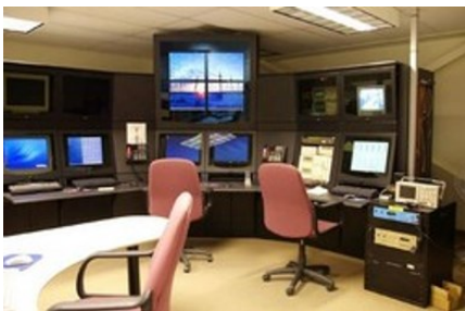
Inside the HAARP control room.
